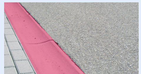
Cart wheels placed in the road gutter area shown in red above - do not place in the driveway or in landscape. If community has no gutter area please ensure a 3' margin from all landscape and fixed items as reflected above.
